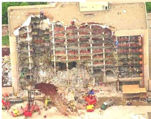
Alfred P Murrah Building, Oklahoma City, Oklahoma, Apr 19, 1995: Progressive collapse extended damage beyond that caused directly by the bomb.
